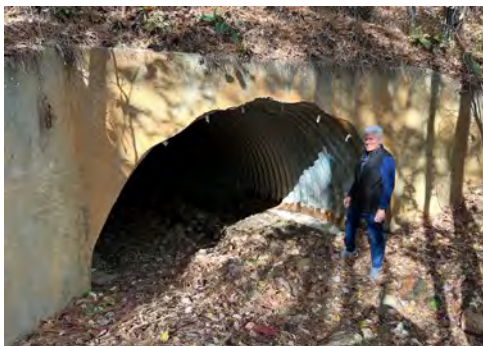
▲ Board liaison John Nettuno inspects the large culvert under Balsam Drive after work was complete repairing and reinforcing the culverts running beneath Balsam and Bonneset. The culverts were one of nineteen major projects completed in 2024 by the MRC. Footings along the sides were replaced, a new channel was centered to keep water away from the footings, and the endcaps were shored up where the slopes were washing away.
